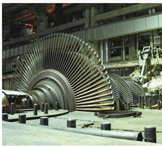
▲ A turbine in a power station being repaired. The turbine is about 5 m across
